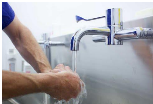
Fig 2. Hand wash sinks should be lever or sensor operated and not have a plug or an overflow
